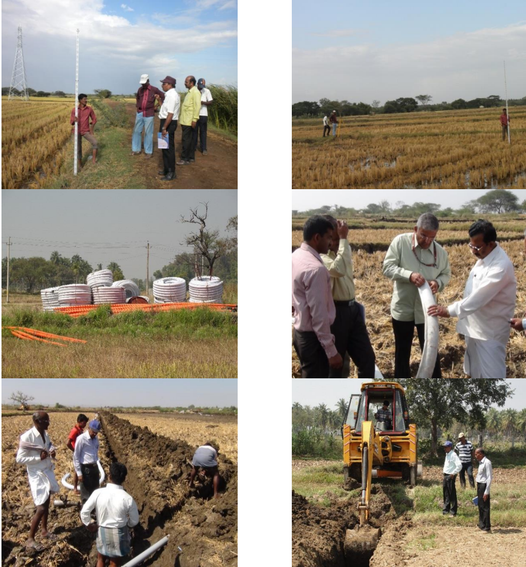
A general view of survey work and installation of sub surface drainage pipes at Tyavanagi village
